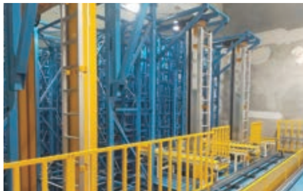
Automated Storage & Retrieval System
